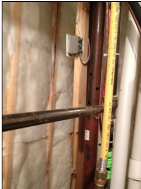
14. Continuity not verified
